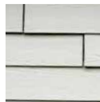
Gaps in Fiber Cement
