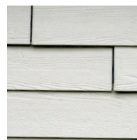
Gaps in Fiber Cement
